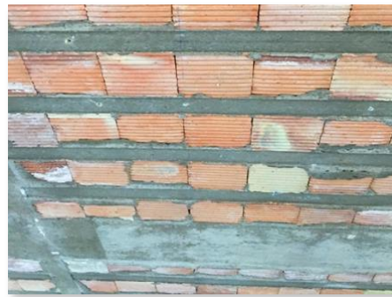
9 Millbank: potted slabs before treatment
