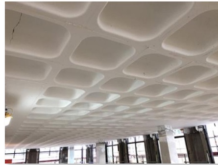
Echo building: waffle slabs protected with AITHON A90H
